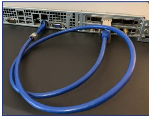
Figure 14 Cat-5 cable (connected to SFP and server)
